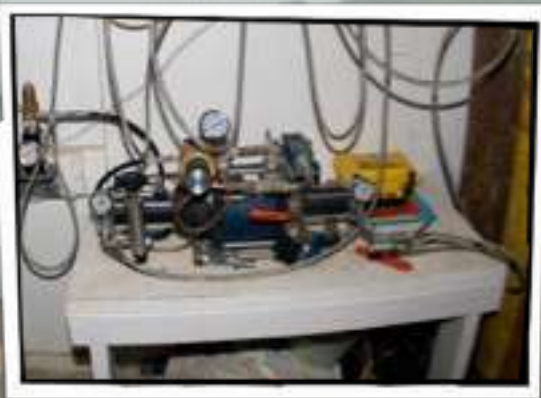
2 x Haskel Booster pumps
